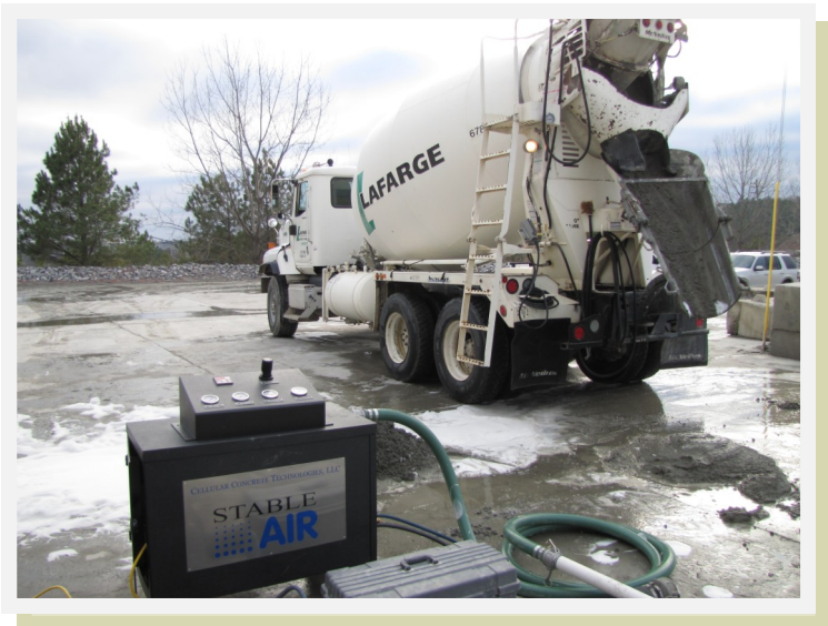
Cement truck and Cellular Concrete Technologies Model 300 machine on job site preparing Flowable Fill.
